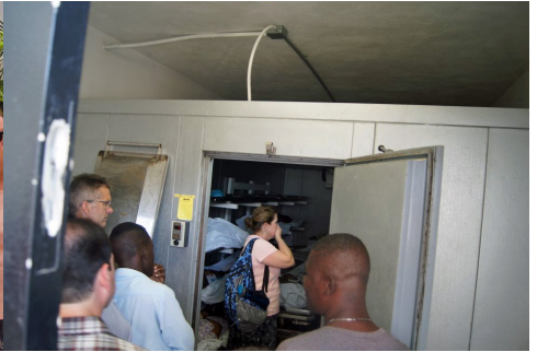
bad smell in morgue cold room
