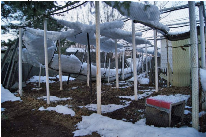
Snow collapsed the rear wire mesh roof.
