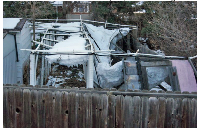
10 foot wide, 40 foot long, roof collapse on right
